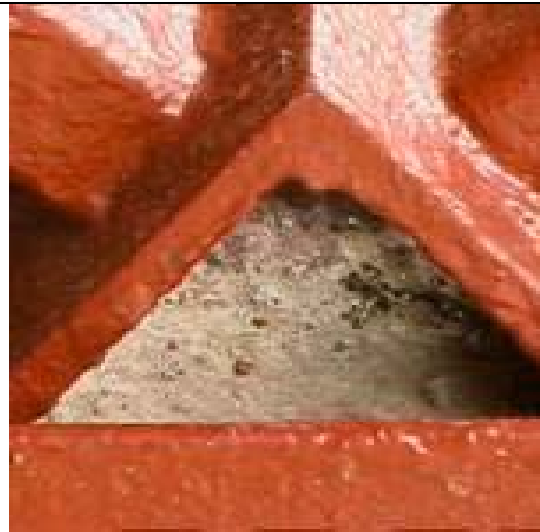
Fig. No. 18. Poor design, where water and contaminants are retained, without a drainage hole.
