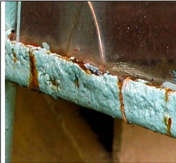
Fig. No. 17. Cavity where water and contaminants are retained and due to oxidation the glass breaks.
